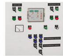
Control panel of a supply inverter with automation control unit Cat. N° 26193
